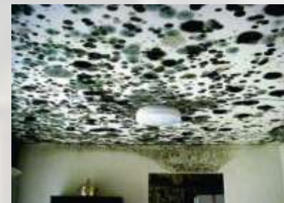
Gambar 1: Kulat di siling (Sumber: http://ocsjanitorial.com )
