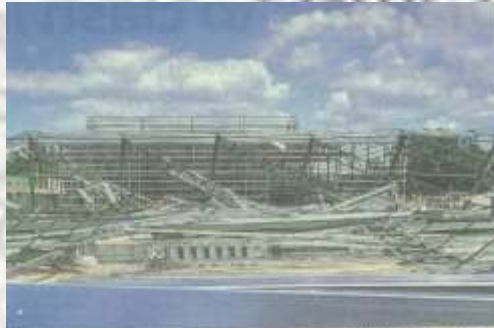
Tragic accident: The metal structure of the construction site that fell on the workers at the Bukit Kemuning industrial area in Rawang. — Bernama
