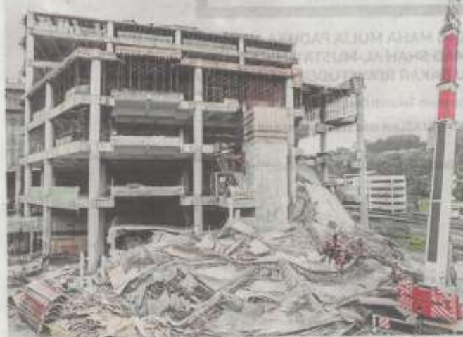
The multistorey car park construction at the Gombak Putra LRT station in Jalan Akhbar, Kuala Lumpur.
