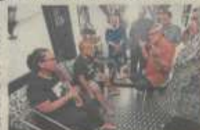
Giving 'freak' lift a safety check, Khalid said the forensic report by DOSH on the cause of the lift incident would be ready by Aug 16. It is believed that the fail-safe protection brakes, which should have kicked in when the car speeds more than usual, ceased to work when the lift fell from the fifth floor of Block C.
