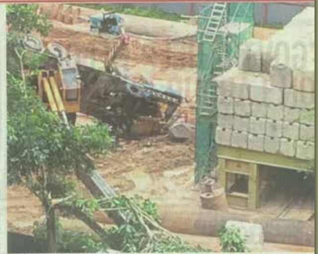
The crane was being used to lift stone slabs in Taman Desa, Kuala Lumpur, yesterday, when it heeled over. PIC COURTESY OF FIRE AND RESCUE DEPARTMENT
